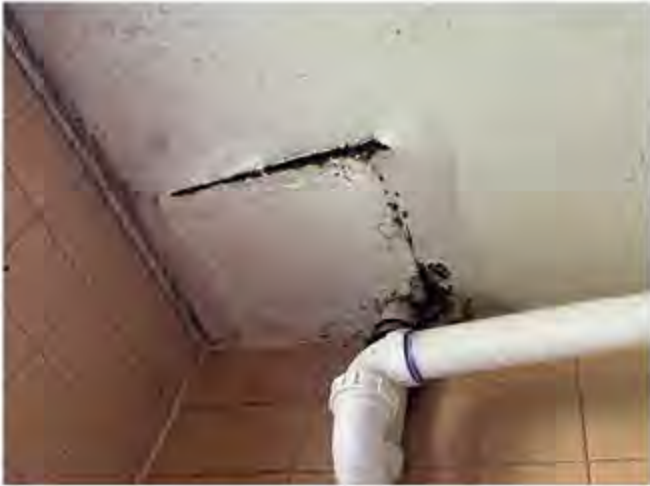
Lack of ventilation creates bathroom ceiling issues.
